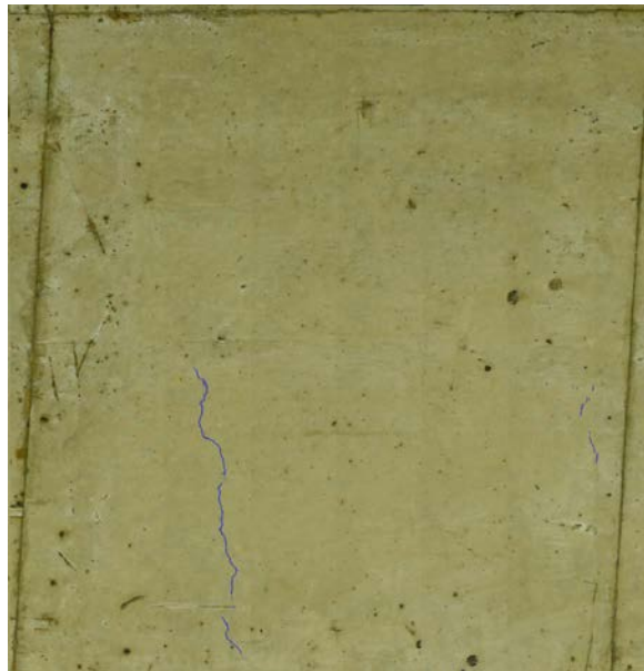
Fig. 12. Result of automatic crack detection
